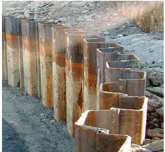
Steel Retaining Wall
